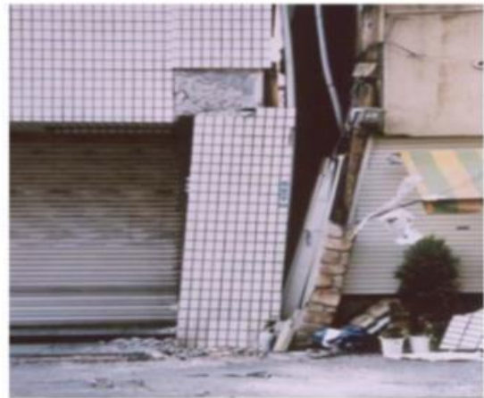
Figure1.10. Joint parasismique insuffisant
