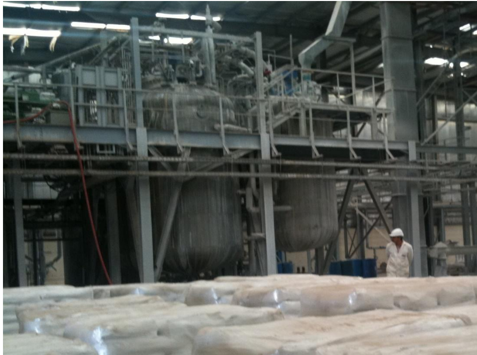
Figure I.13 : Station production silicate de soude
