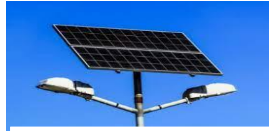
Figure III.9 : luminaire LED solaire
