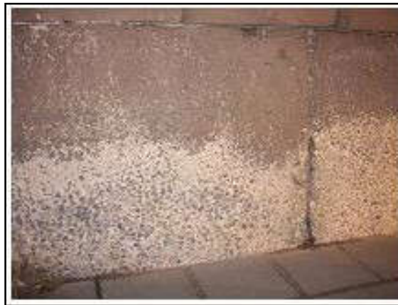
Figure I-12 : Écaillage de surface. [1]
