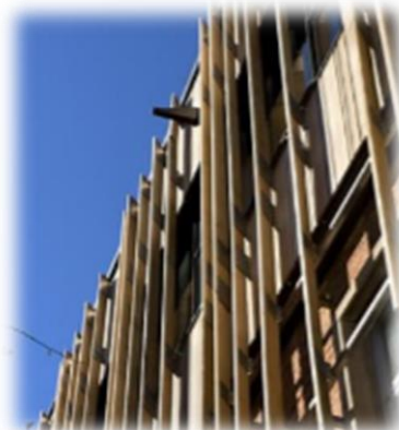
Figure 18 les stores vertical 27
