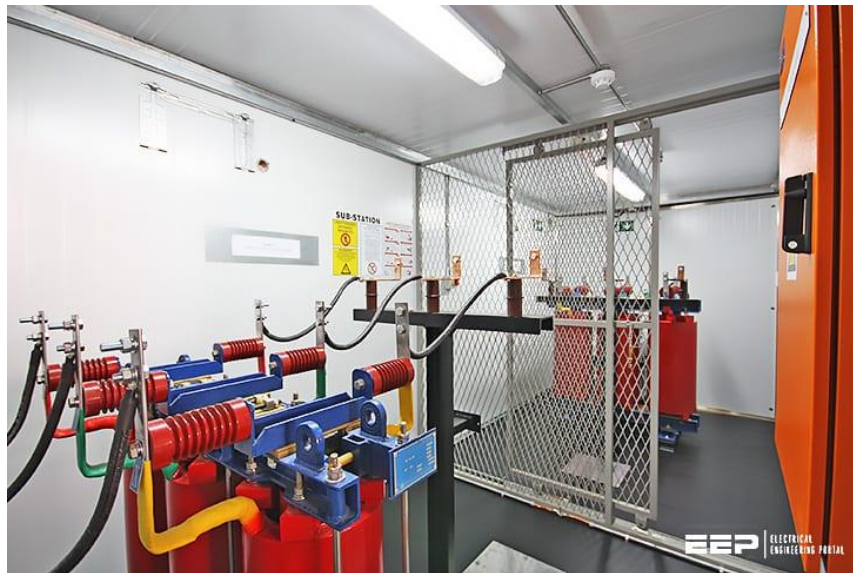
Figure 1. 20:Dry type transformer
