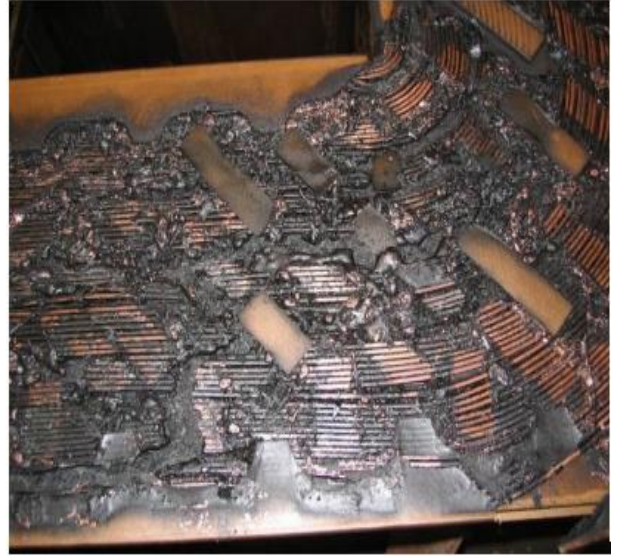
Figure 2. 5:Short-circuit between turns
