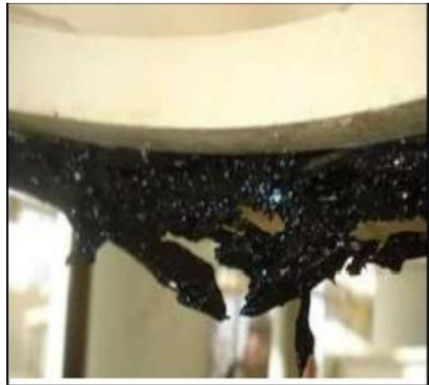
Figure 2. 1:Leaks of joints
