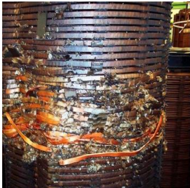
Figure 2. 4:Overheating of a winding
