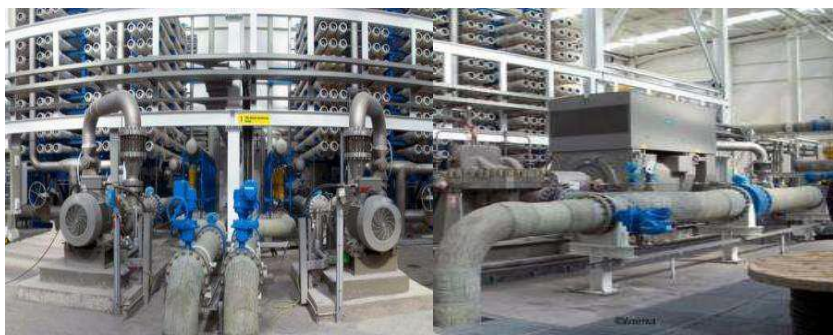
Figure II.10: Pompes BOOSTER Figure II.11: Pompe à haute pression
