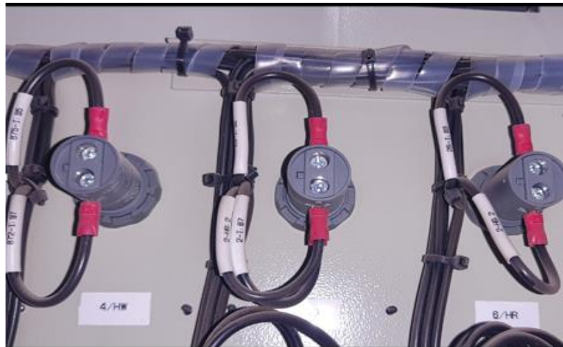
Picture IV.18 : Indicators of MV feeder's status back side wirin
