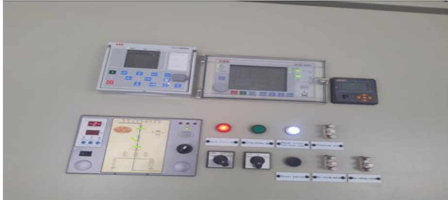
Picture II.12 : Control panel of the bus coupler switchgear in pellet plant 34.5/6.6KV Tosityali -Algerie.
