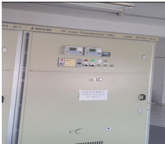
Picture II.17 : 2#main transformer electrical switchgear in Pellet substation tosyali-algerie .
