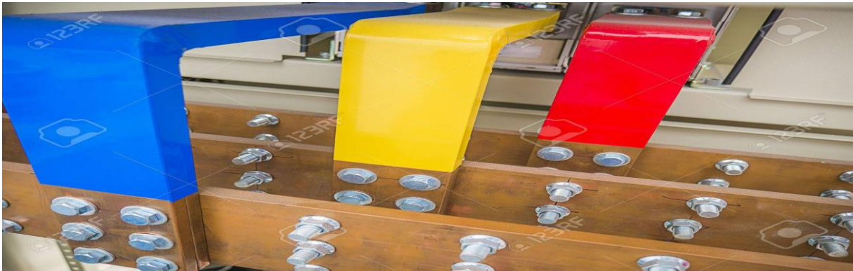
Picture II.3 : Three phase bus bars in electrical panel.
