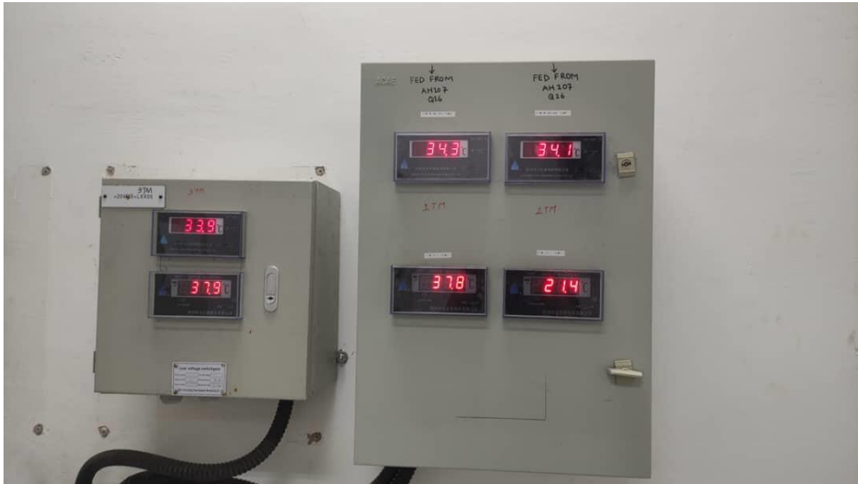
Picture III.8 : Periodic monitor panel of main transformers 34.5/6.6KV of pellet plant TOSYALI
