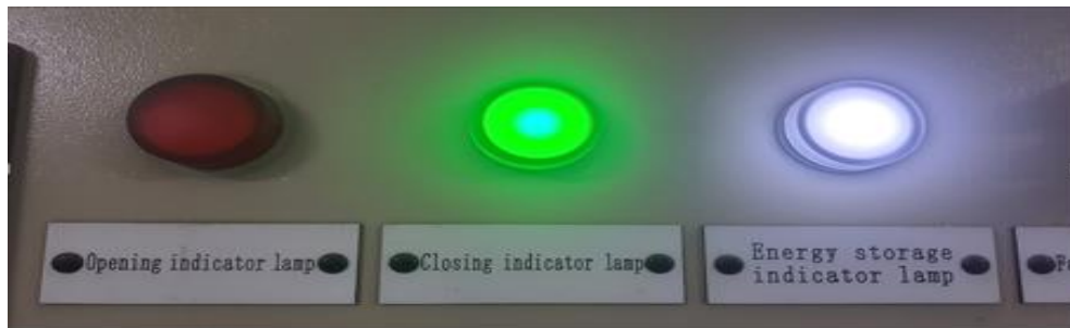
Picture IV.17: Indicators of MV feeder's status
