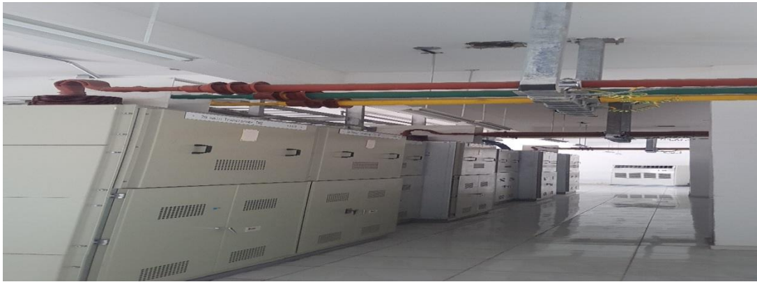
Picture II.16 : Back side of 34.5KV switchgear in main substation into the transformers in pellet plant 34.5/6.6kv Tosyali-Algerie
