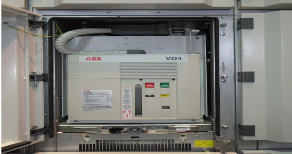
Picture II.19 : A forward picture of one VCB in pellet plant MCC Tosyali-ALGERIE.
