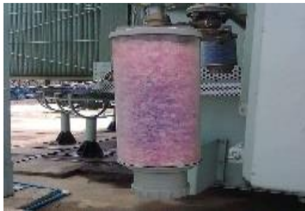
Picture III.13 : silica gel bottle installation in the transformer before use and after the expiration date
