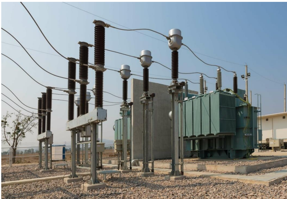
Picture III.11 : Floor of HV substation full by stones.
