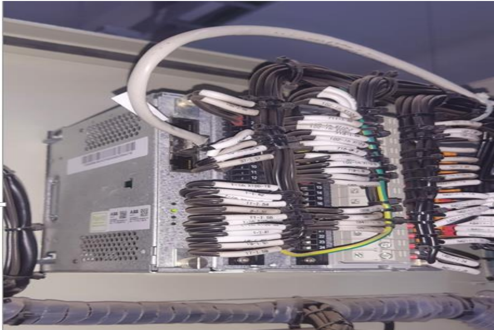
Picture IV.14 : Ref615 backside wires connection place
