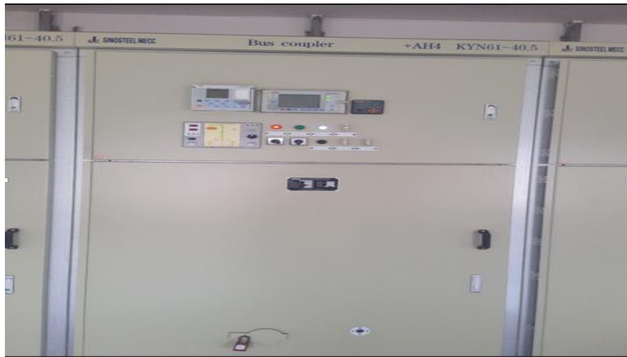
Picture II.10 : Bus coupler switchgear in pellet plant -TOSYALI-ALGERIE
