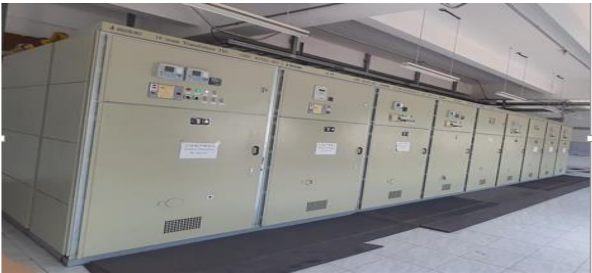
Picture II.1 : Pellet plant substation main power MCC-TOSYALI-
