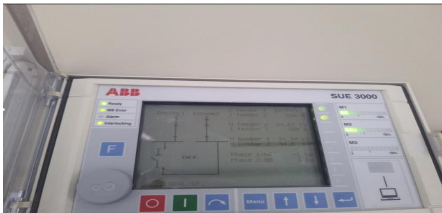
Picture II.13 : High speed transfer device ABB SUE 3000 HMI in pellet plant substation .
