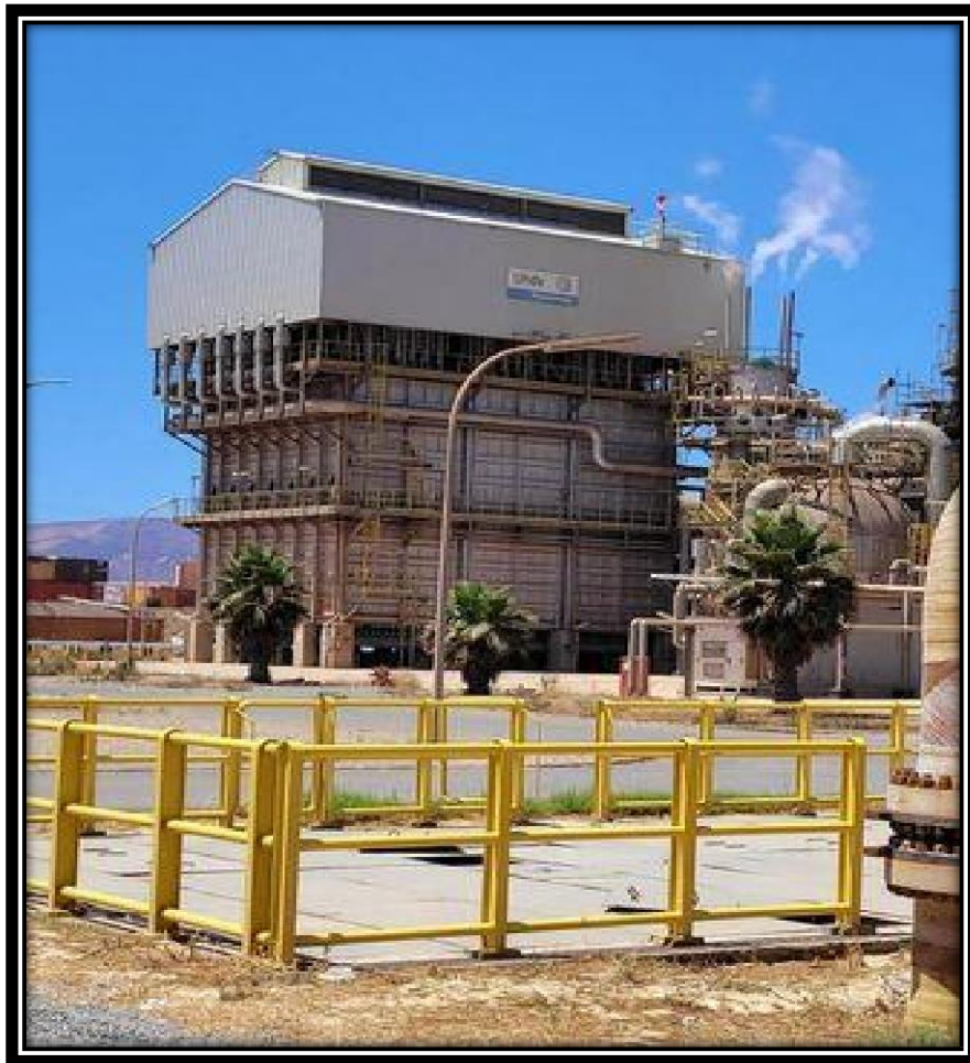
Figure II.1: Reformeur primaire 103B001
