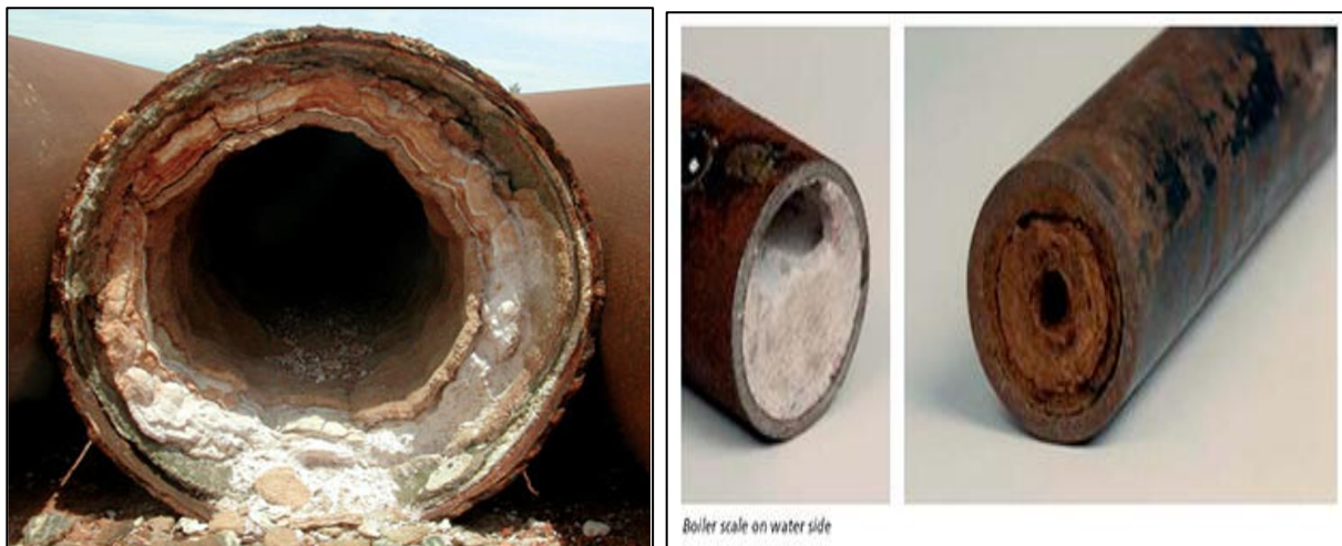
Figure III.2. Entartrage des chaudières
