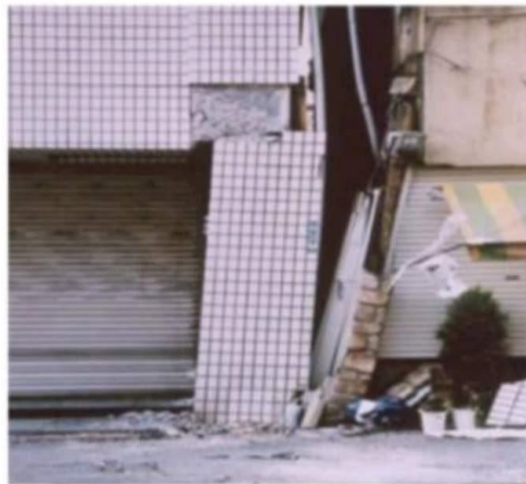
Figure 12: Joint parasismique Insuffisant
