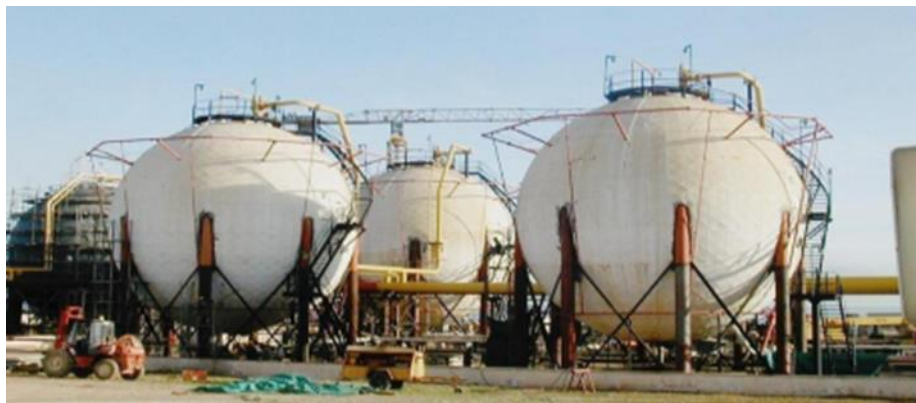
Figure I -5:Sphères de stockage
