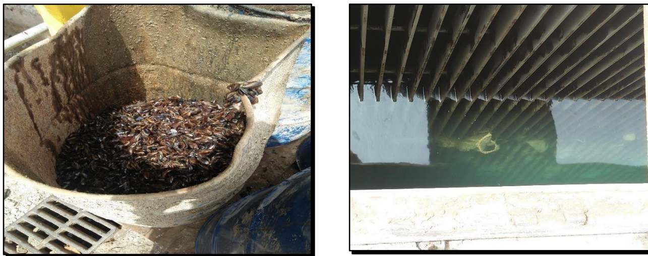
Figure III-13 Colmatage des installations
