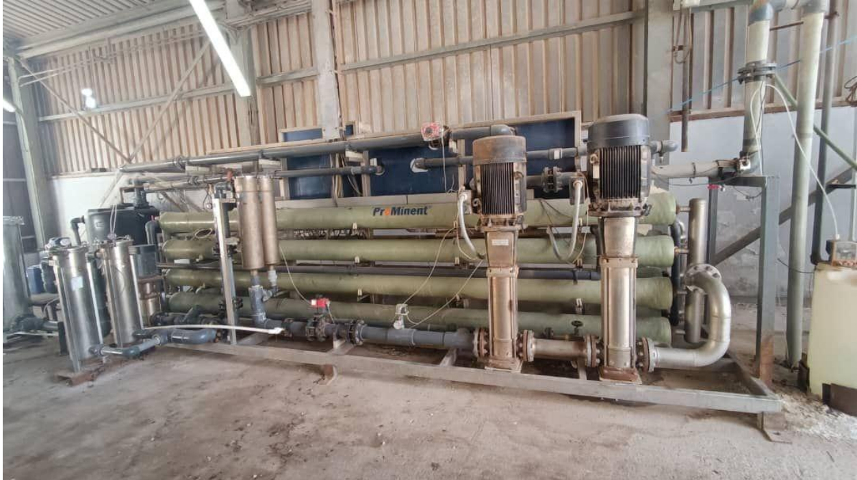
Figure 4: Reverse osmosis unit at Adwan Chemicals
