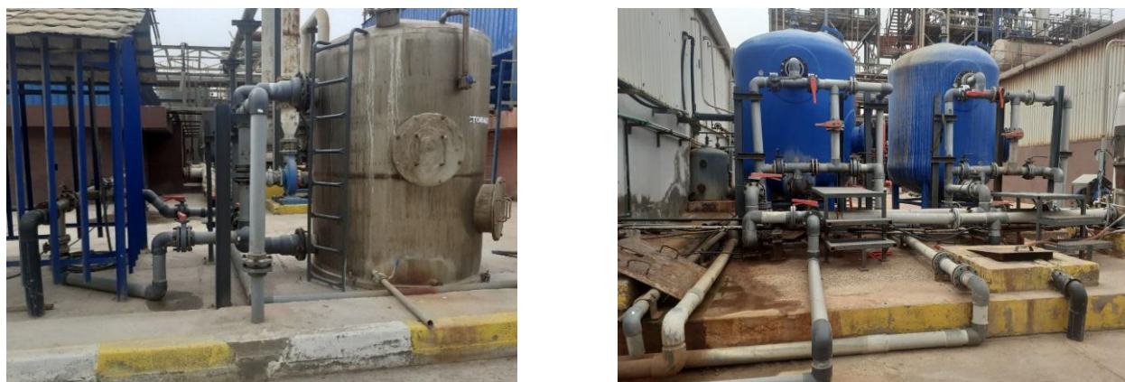
Figure 2: Sand filters at Adwan Chemicals' water treatment plant
