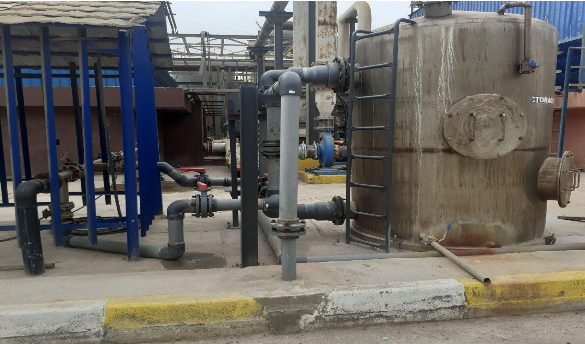
Figure 8: Newly added sand filter at Adwan Chemicals water treatment plant
