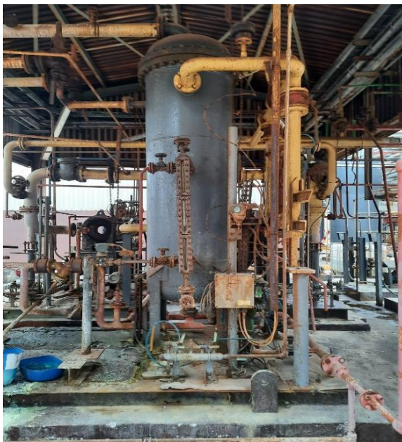
Figure 3: Separator at Adwan Chemicals
