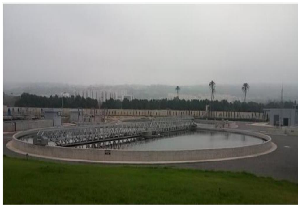
Figure II.4 Décantation secondaire (clarification)
