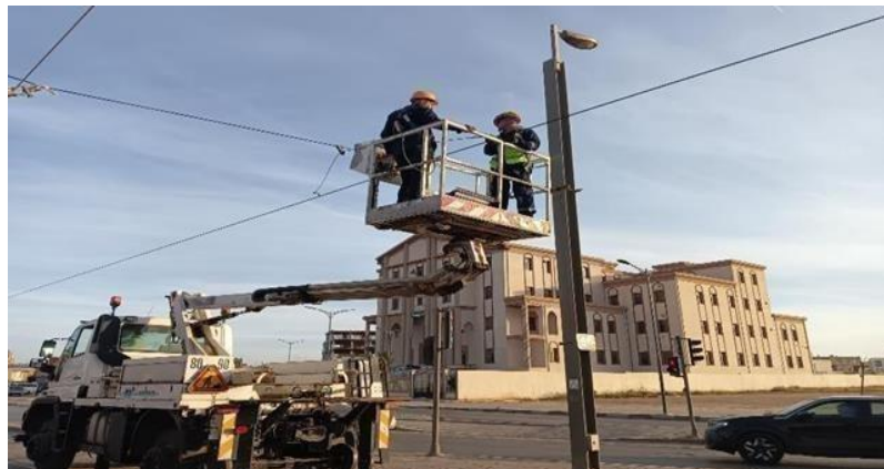
Figure I.5 : La maintenance de SETRAM.
