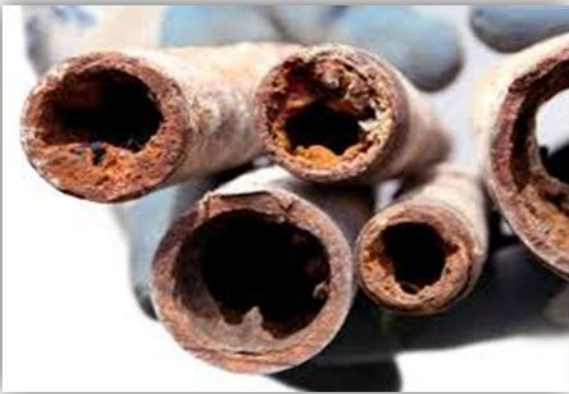
Figure 16: Corrosion des canalisations [31].
