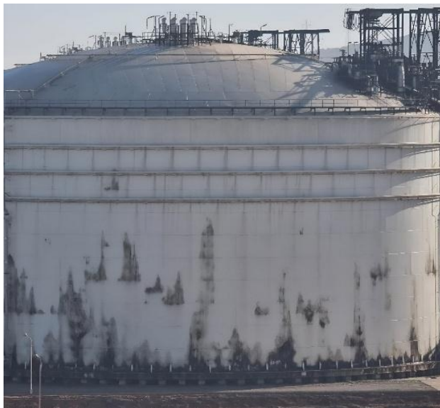
Figure I. 6: Bac de Stockage
