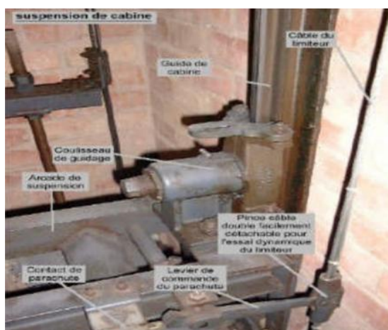
Figure I- 5 : Suspension de cabine.
