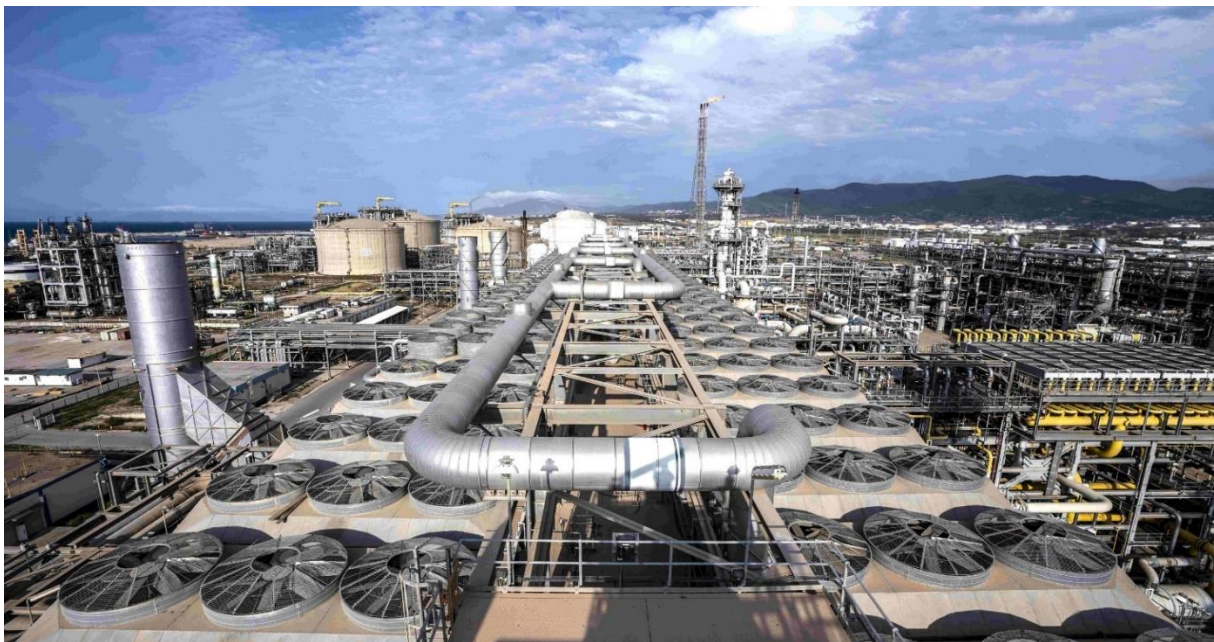
Figure 3 Close-up of the Fin-Fan Air Coolers [6]
