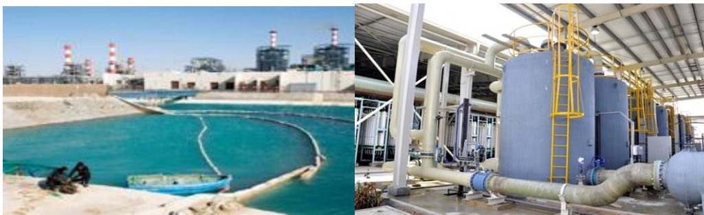
Figure 10 : Station de dessalement
