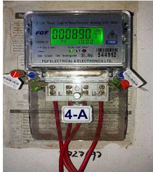
Figure 3.4: Smart card prepaid electric meter
