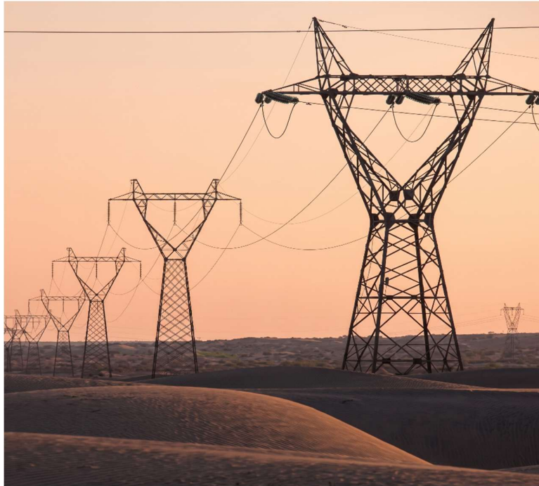
Figure1.1 : high-voltage power line
