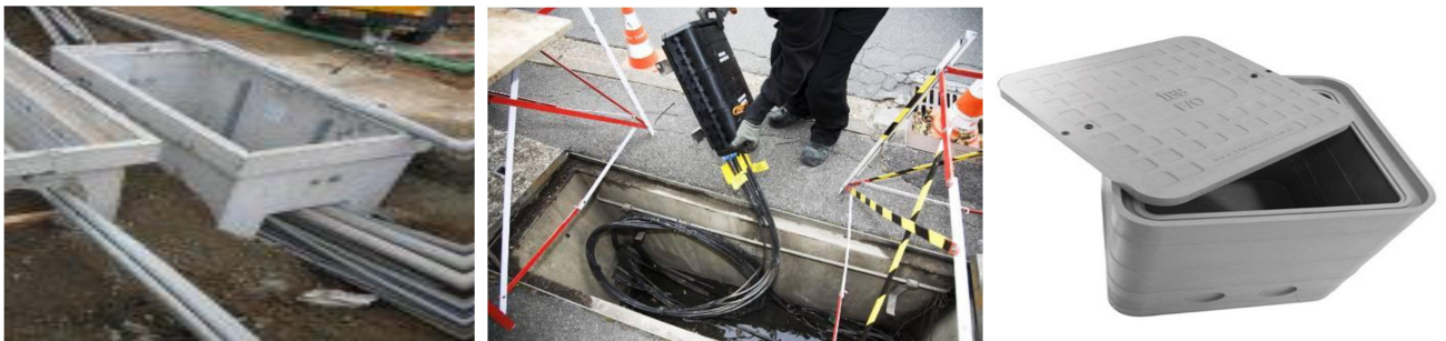
Figure 4.16 : Chambre A2. Figure 4.17 : Chambre A3. Figure 4.18 : Hand hole.
