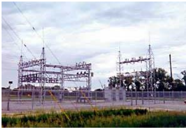
Figure I- 8: Poste de Distribution
