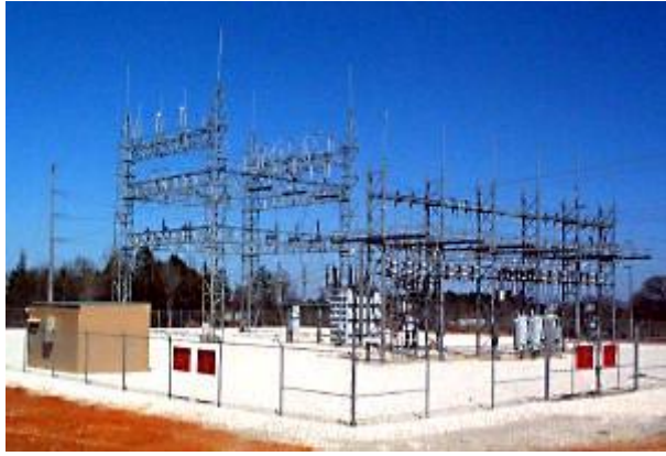
Figure I- 6 Sous station de distribution
