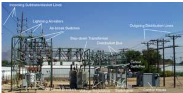
Figure I- 9: Sous-Station de Distribution
