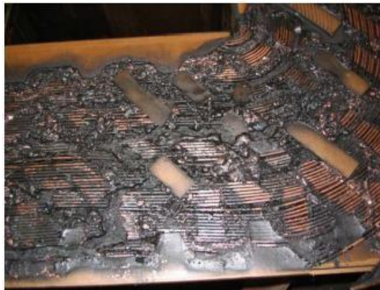
Figure II.4 :Court-circuit entre spires
