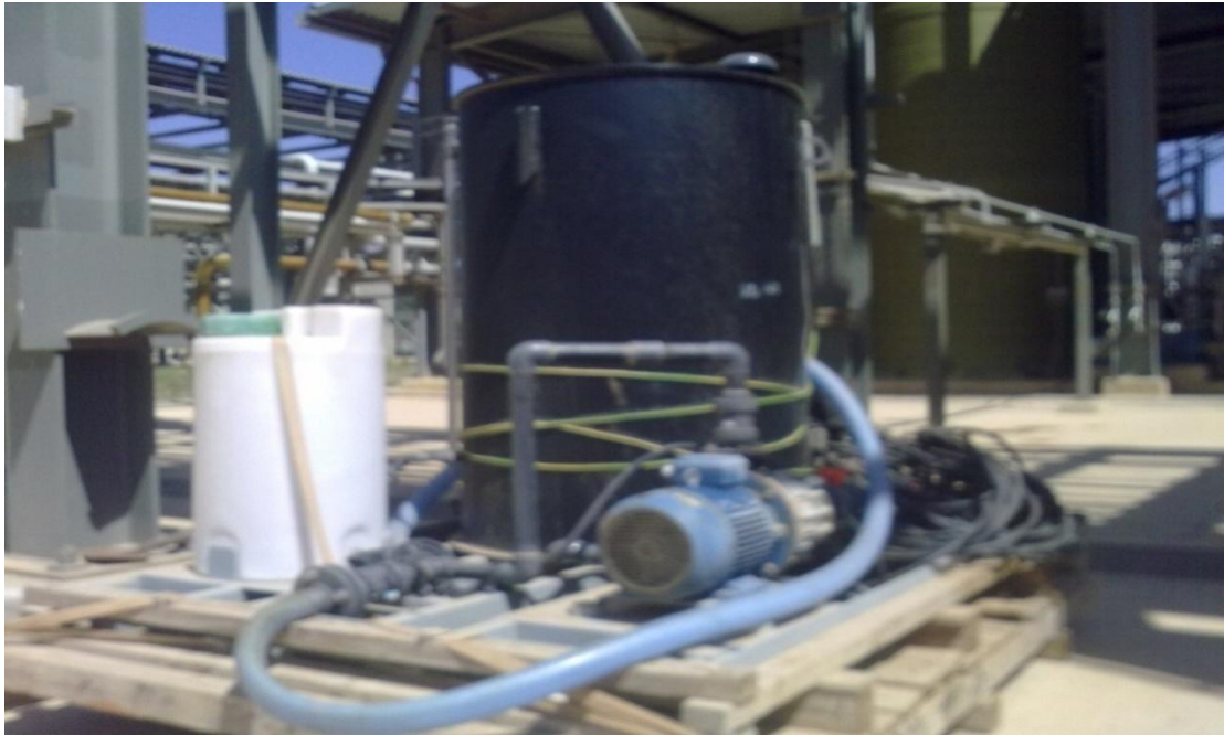
Figure II.10: La station mobile de lessivage ‘skid acide ‘
