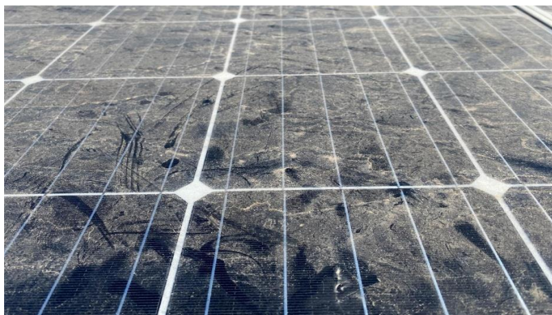
Figure 11: Non-uniform dust distribution on solar panels [13]
