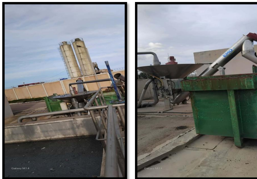
Figure II.5 Clarificateur de sable
