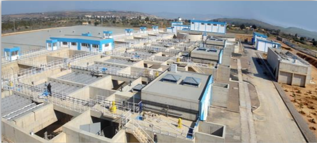
Figure. III. 4. Station de traitement de l'eau potable de SIDI LAHDJEL
