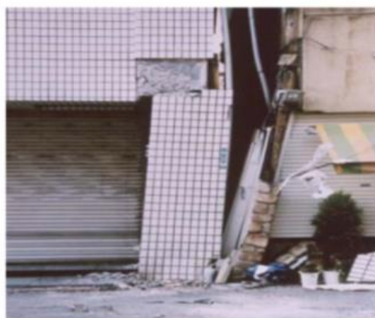
Figure I.13. Joint parasismique insuffisant
