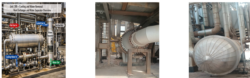
(a) P.Overview of U.300 – (b) Front View of the Heat (c) Side View of the Heat Ex- Cooling and Water Removal. Exchanger. changer.
