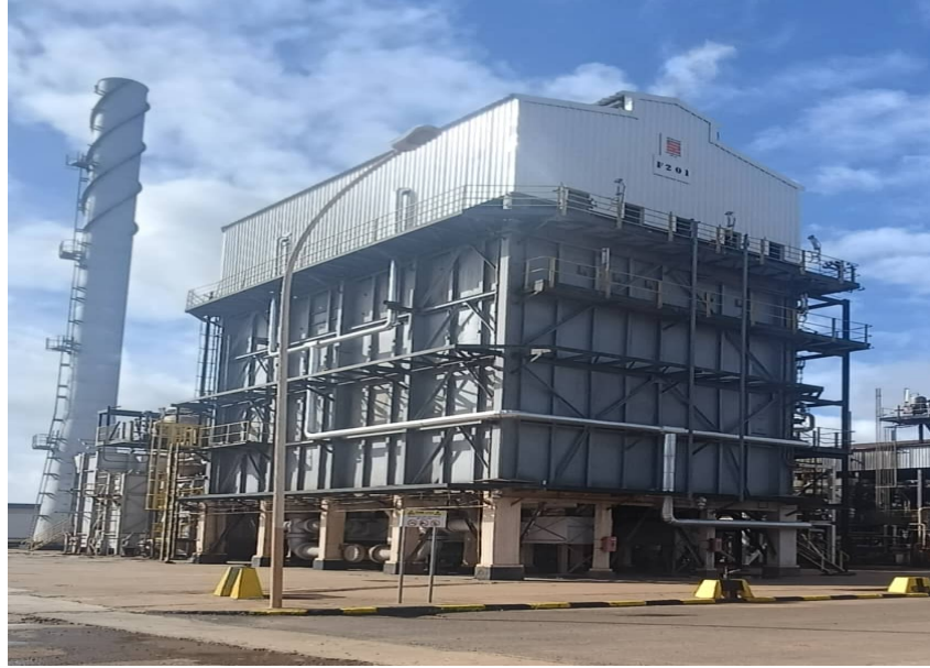
Figure 1.6: Reforming Furnace in Unit 200.
