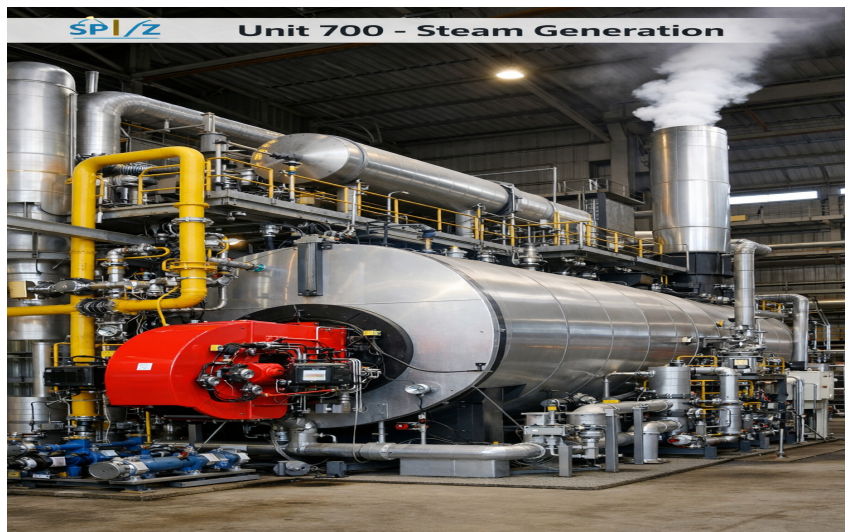
Figure 1.11: Steam Generation Unit.
