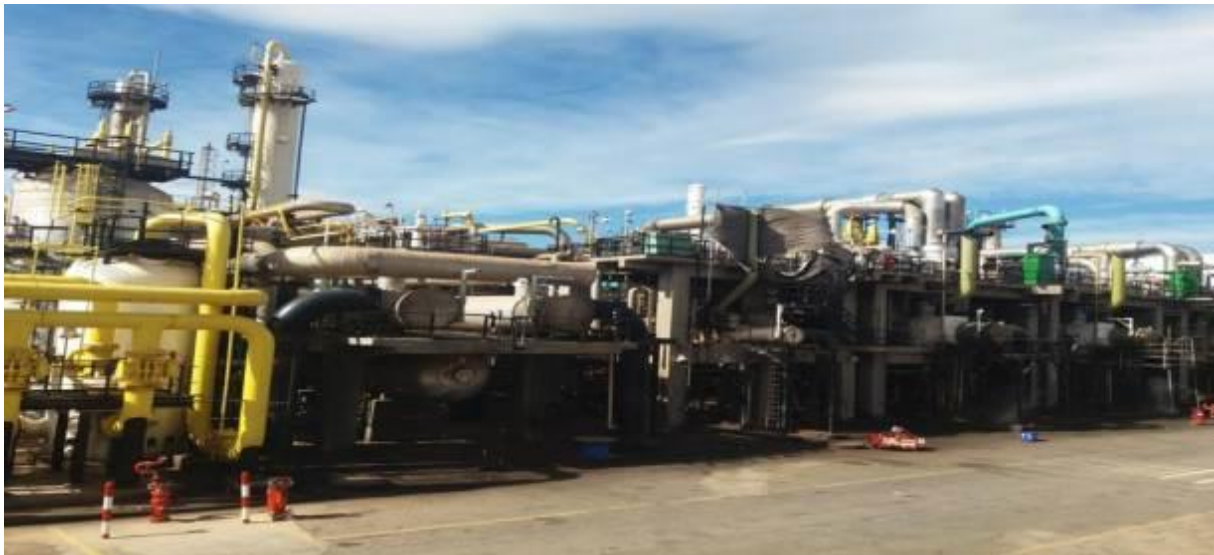
Figure 2: Zone de processus du GNL1/Arzew.
