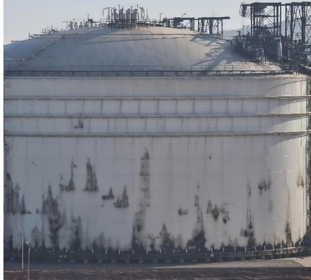
Figure I. 6: Bac de Stockage
