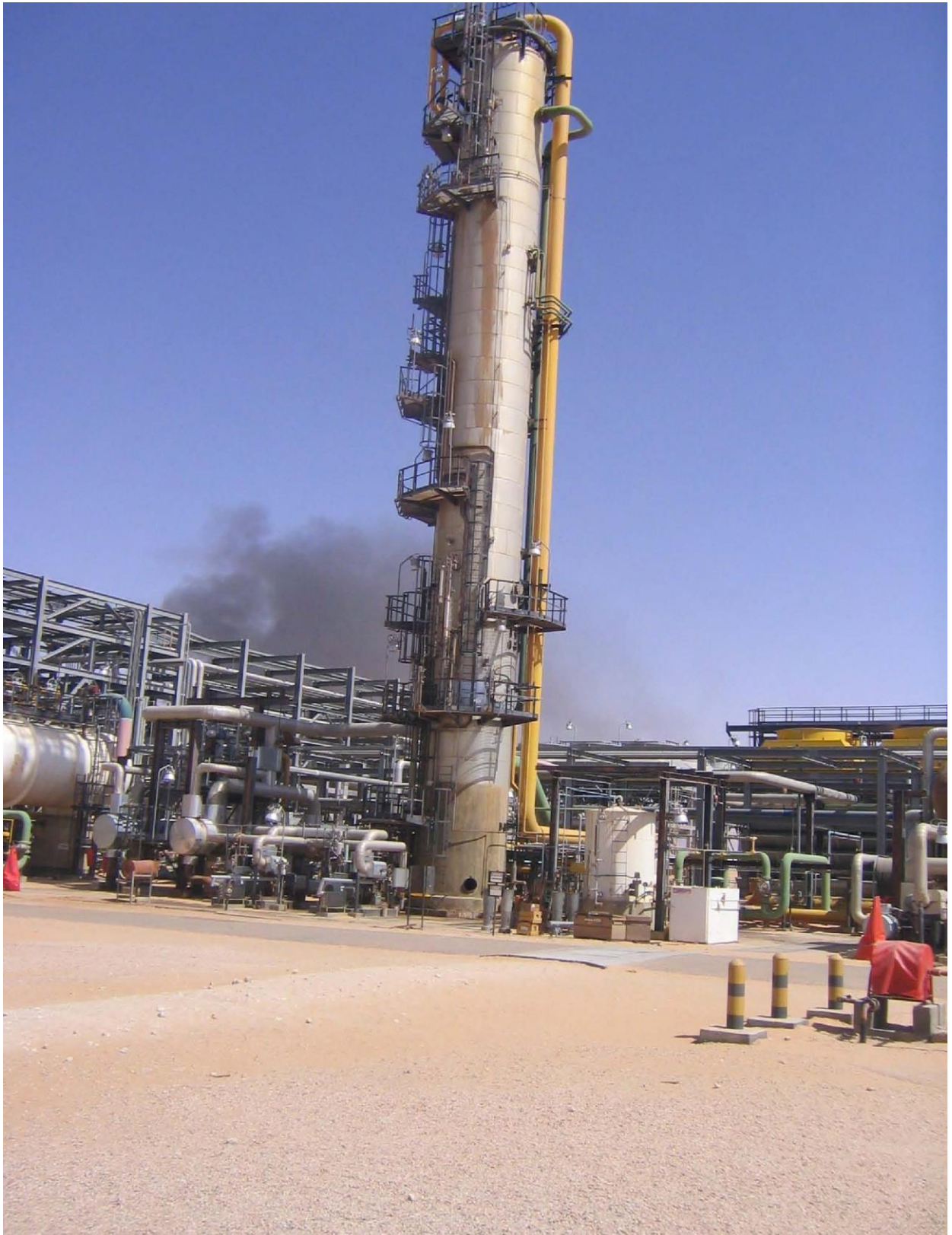
Figure II. 3: La colonne de stabilisation DA-4501.
