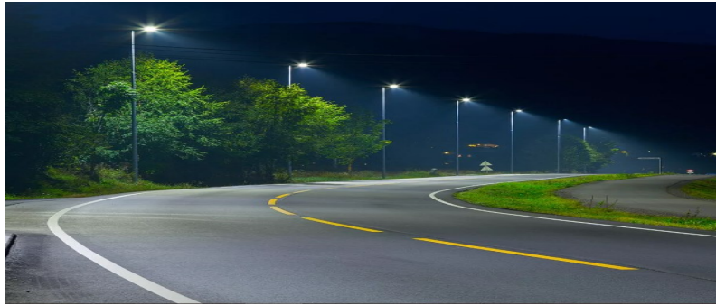
Figure 2 : Luminaire public intelligent [9].
