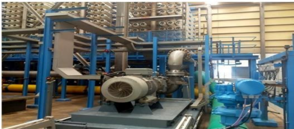
Figure II.12: la pompe Booster
