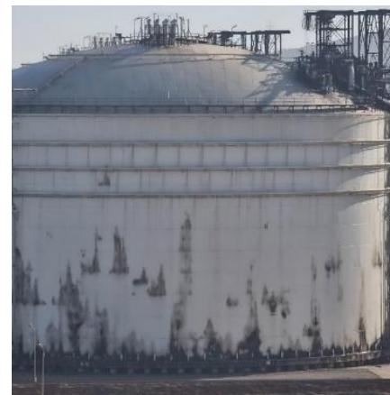
Figure I. 7: Bac de Stockage
