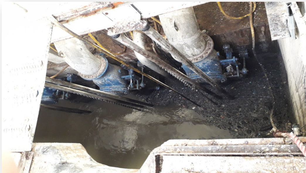
Figure n°15: Station de relevage des eaux brutes
