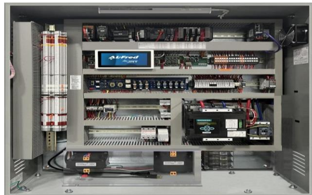
Figure 24: Automate Programmable Industriel [32].
