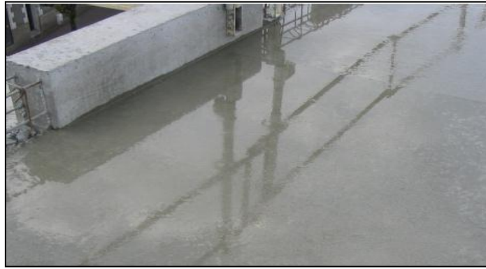
Figure 2.2: Ressuage du béton
