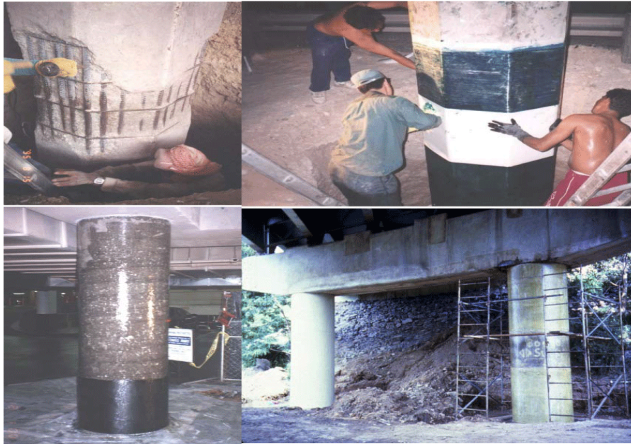
Figure 16: Repair and rehabilitation of corroded bridge & RC columns with FRP Composites (Mosallam, 2014).
