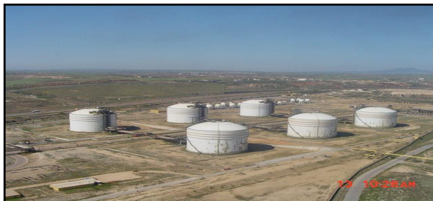
Figure I.4 bacs de stockage.
