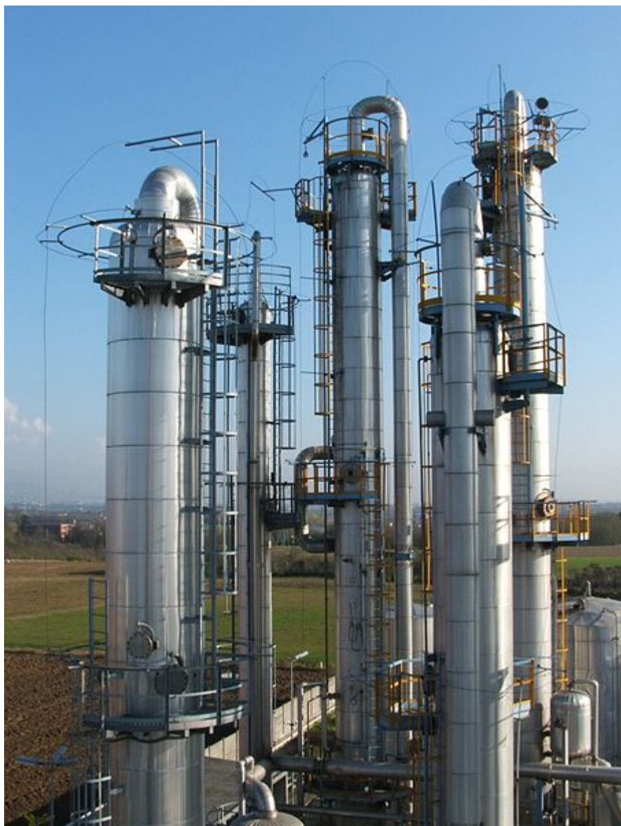
Figure I.5. Colonnes de distillation industrielles.
