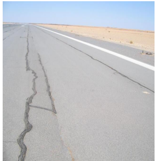
Figure 4.2 : Fissure de joint
