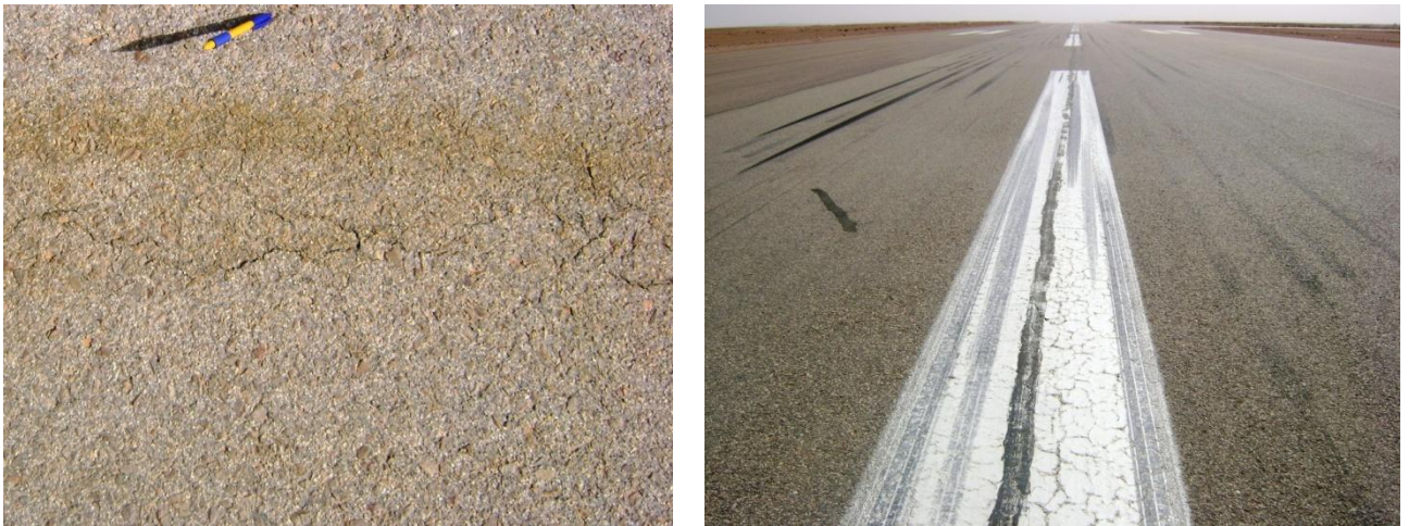
Figure 4.9 Fissure de fatigue
