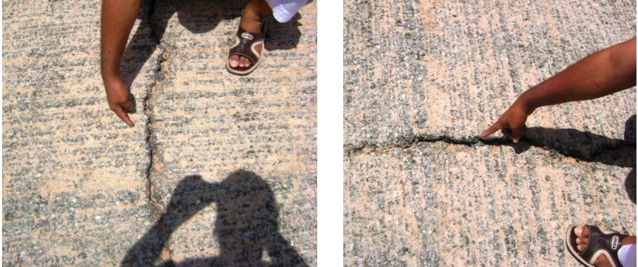
Figure 4.5 Fissure de fatigue
