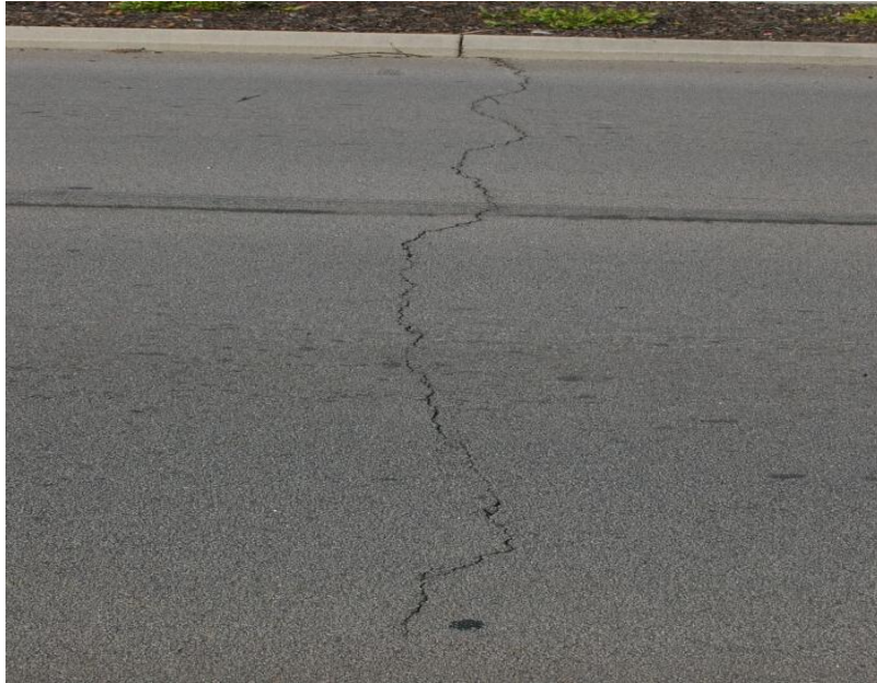
Figure II.12 : Fissure fine et transversale
