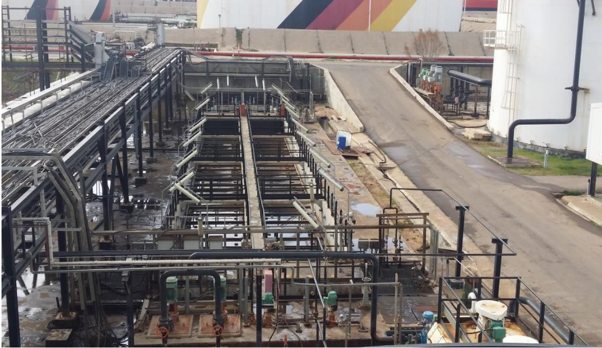
Figure II.15: Zone 27 API Separator
