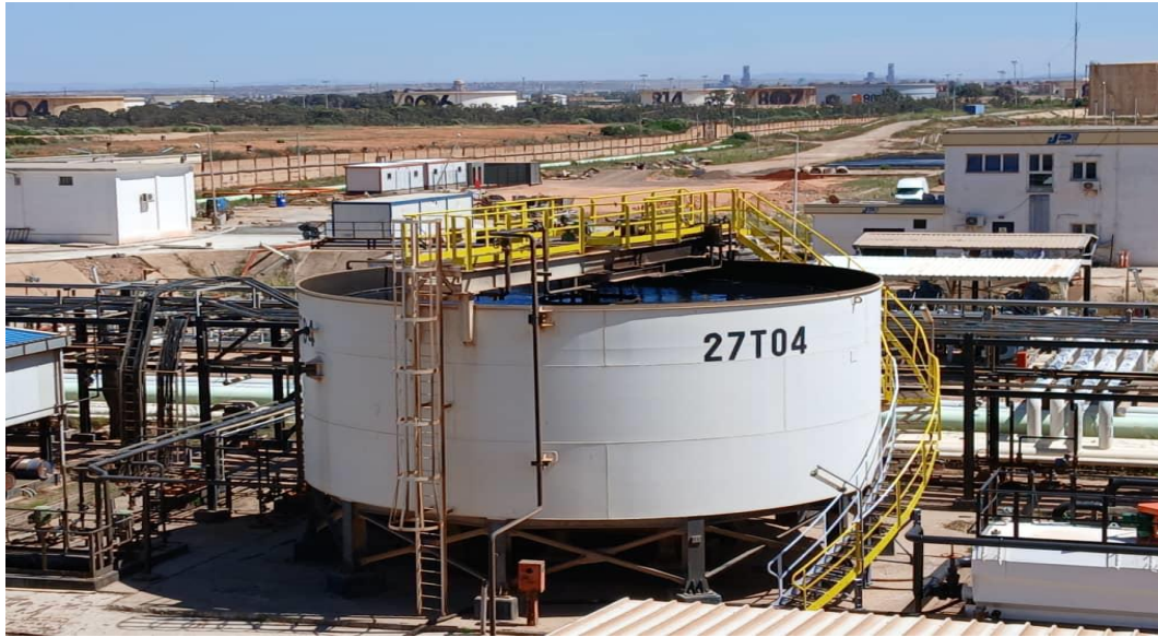
Figure II.20: Sludge thickening or sludge handling section of Zone 27
