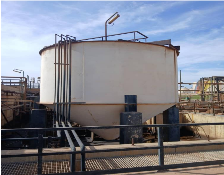
Figure II.11: Sludge thickener of Unit 1800
