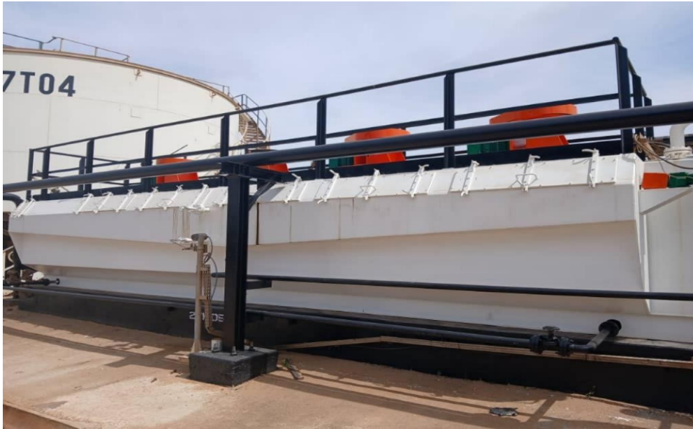
Figure II.16: IGF/EGF flotation unit of Zone 27
