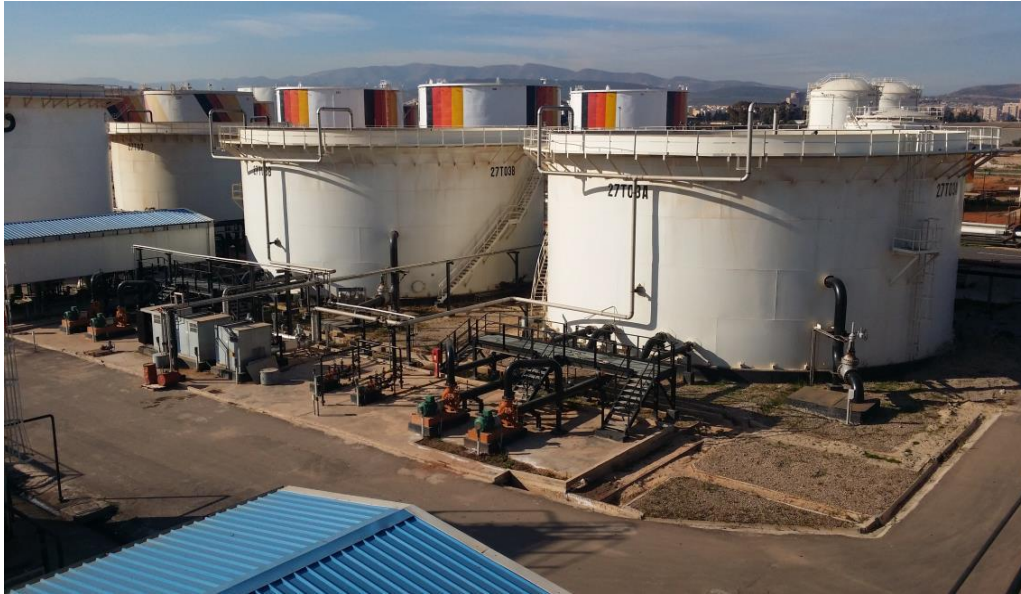
Figure II.17: SBR biological reactor of Zone 27
