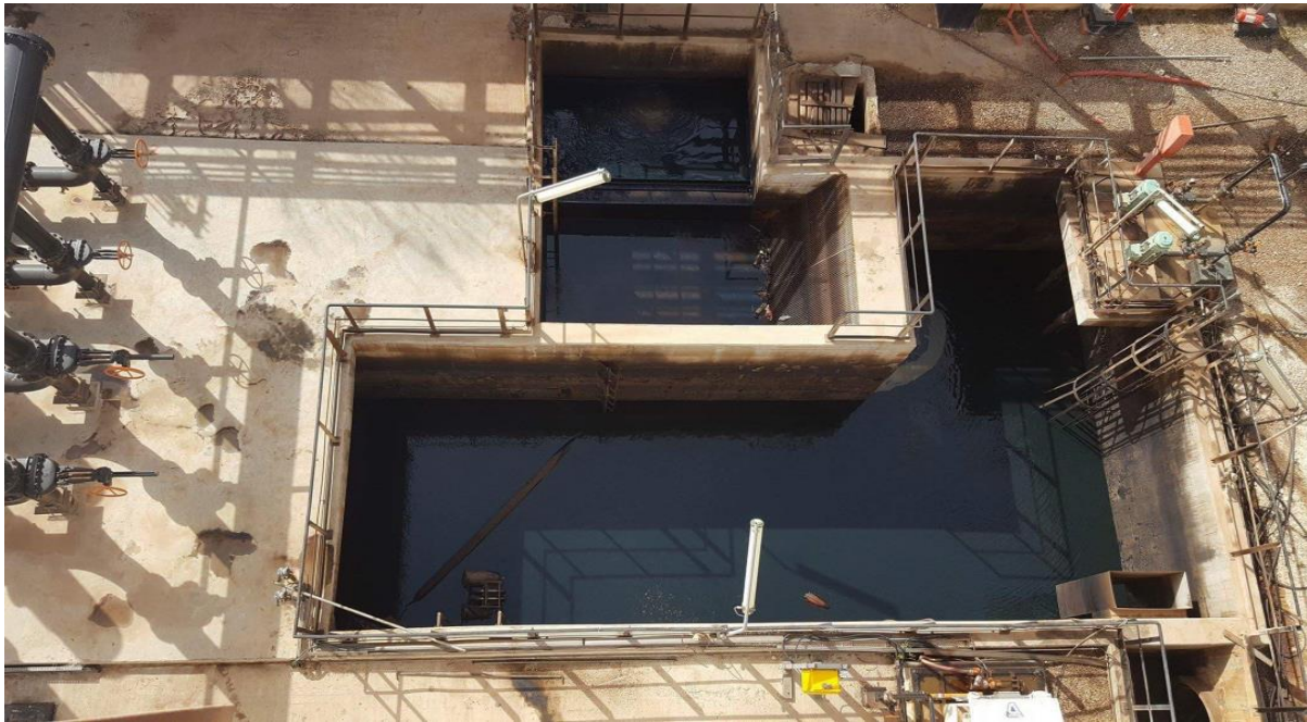
Figure II.14: Stormwater basin of Zone 27
