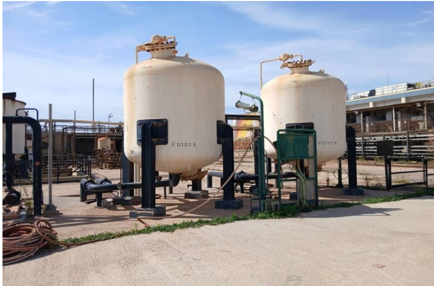
Figure II.10: Sand filtration system of Unit 1800
