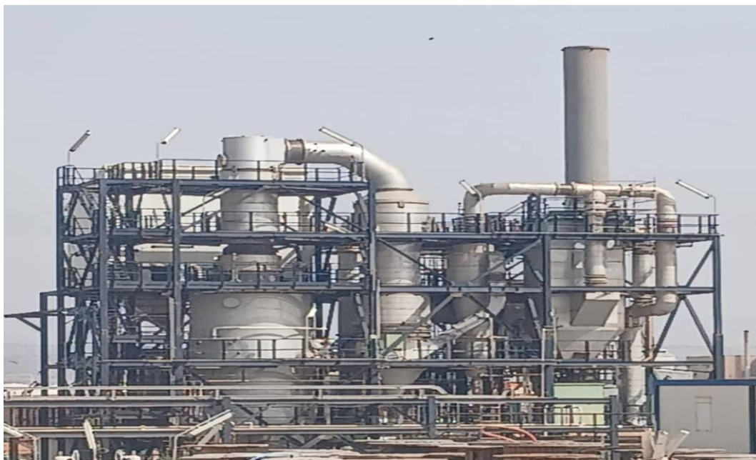
Figure II.21: Sludge incinerator of Zone 27
