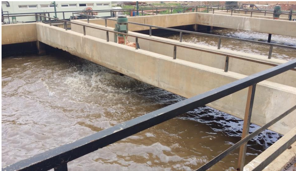
Figure II.9: Biological treatment basin of Unit 1800
