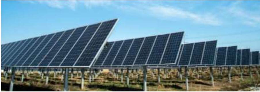
Figure 1: Panneaux solaires photovoltaïques.
