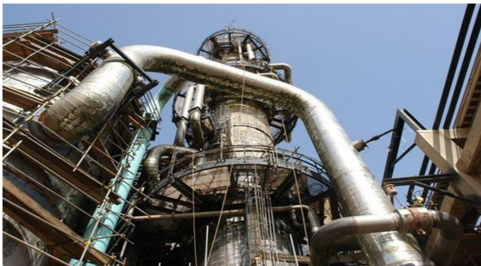
Figure. II.2: L ‘échangeur principal X16C.
