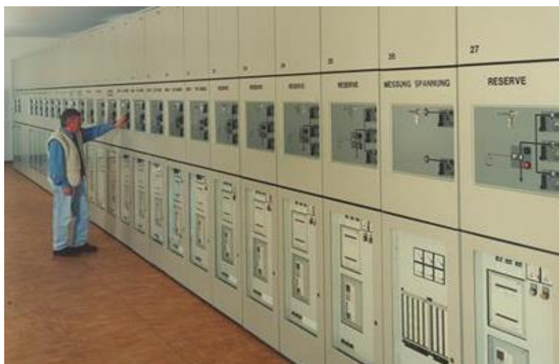
Figure III.20 : Armoire Schneider 5.5kv.
