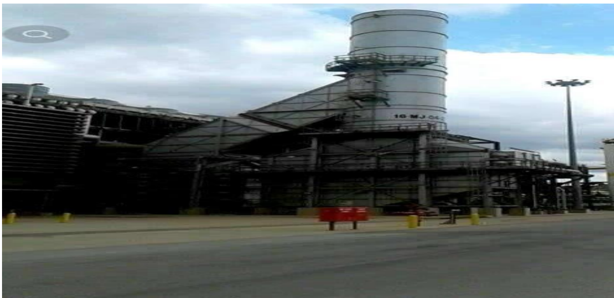
Figure 11: Turbine à gaz fram7 (MS7121E) du complexe GL3/Z
